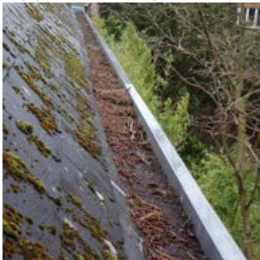
Dak [2]-west: vervuilde goot.
