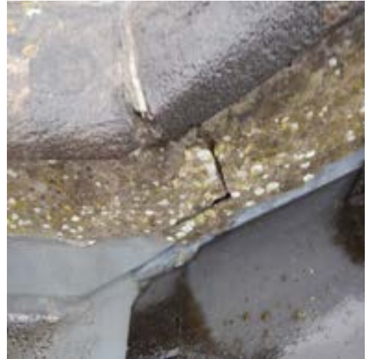
Dak [1]: gebarsten cementering.
