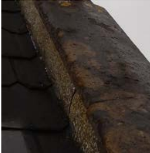
Dak [1]: gebarsten cementering.
