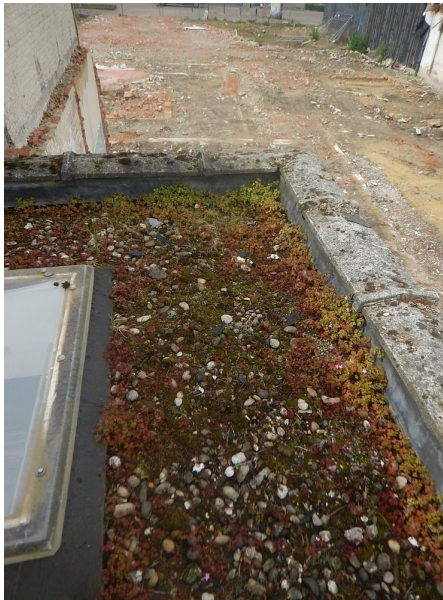
Dak [2]: sterk bemoste ballast.
