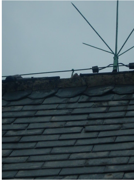
Dak [1]: gebroken nokpan.
